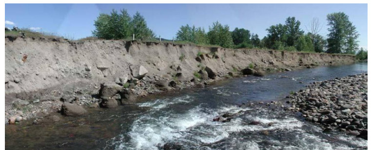
This is an eroding streambank and an unhealthy riparian zone.
