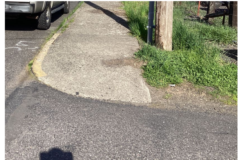
No Detectable Warning Surface
