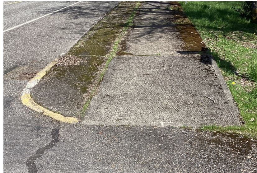
Outdated Diamond Aggregate
